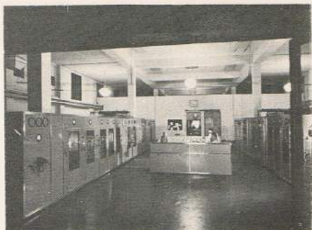
The Transmitter Hall of the British Broadcasting Corporation (BBC) shortwave station at Rampisham. The Hall contains 4 high-powered transmitters and was divided into two by a wall as a precaution during World War II.
