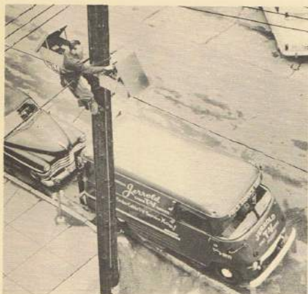
By-passing distribution amplifier with stand-by amplifier in truck permits complete on-pole test of working equipment. Equipped with two-way radio, full test bench, and an emergency power supply, this Dubuque (Iowa) Jerrold CATV system truck is ready for trouble calls anywhere.
