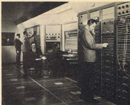
The Master Control Board in the Radio Canada Building in Montreal is the nerve center of the CBC's broadcasting installation. It can handle five transmitter feeds, eight outgoing networks, seven incoming networks, 23 studios, and was designed for one-man operation. The switching of all circuits is performed by remotely-controlled relays.
