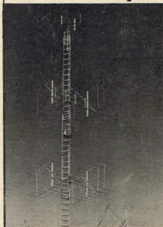
A Typical SITCO Installation
